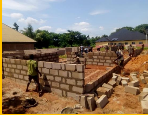
All the labor and sand for the construction at Ohagelode was provided by the community
